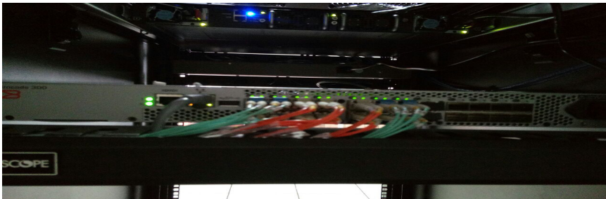
Gambar 18. Sanswitch Data Center
