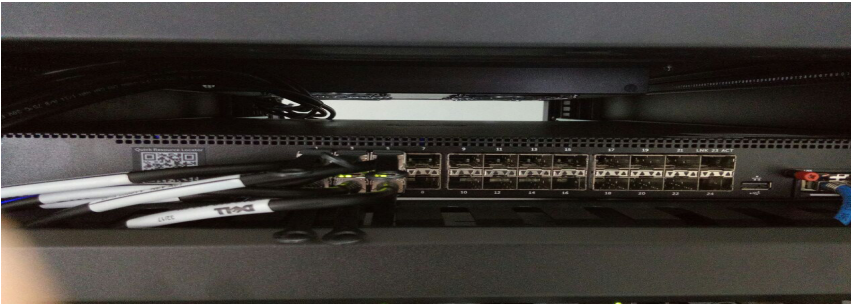
Gambar 17. Data Center Switch
